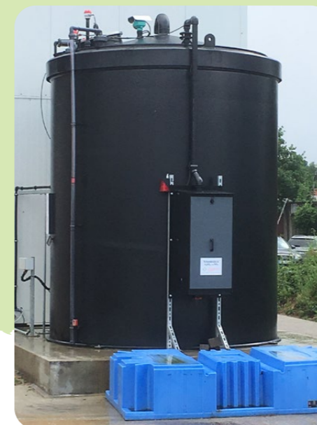
Stationary storage tank
