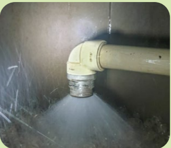
Nozzle in the vapour scrubber
