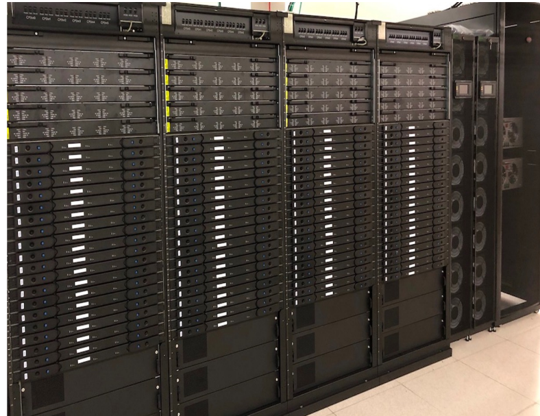
4 racks with 20 blades each (240 computers)
